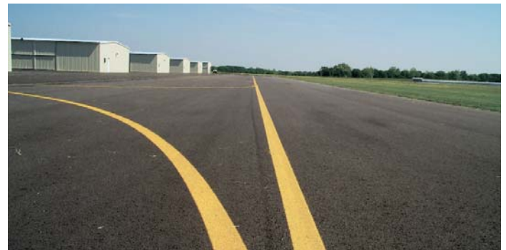
Taxiway markings are yellow. The centerline is a single yellow line, and the taxiway edge is marked by a double yellow line. Dashed edge markings allow the aircraft to cross to the adjoining apron.
